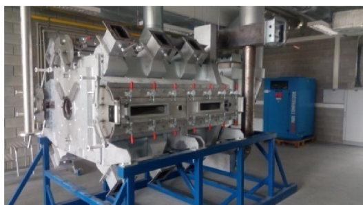
Figure 5 – The appearance of the installation for the combustion of biogas
