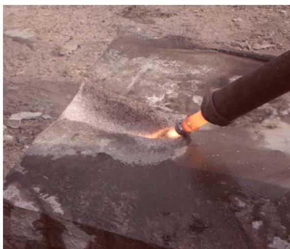
Figure 4 – Formation of slotted working by using BVR60 Thermal cutter torch with gas-dynamic nozzle
