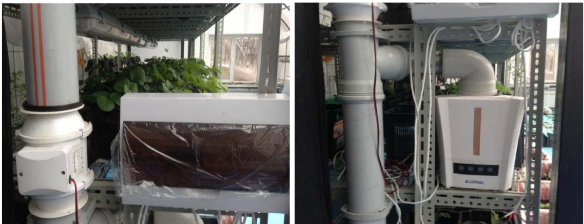
Photo 3 - Gas regulation fan (photo on the left). "Cold steam" and air ionization device and (right)
